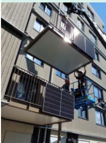
Balconies with PV
