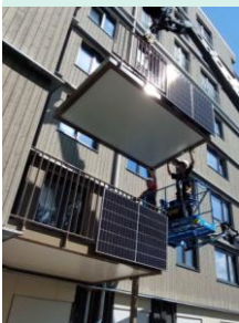
Balconies with PV
